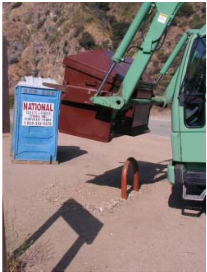
Figure 4—Dumpster being lifted off pipe stand. Pipe stand is set in concrete footings.
